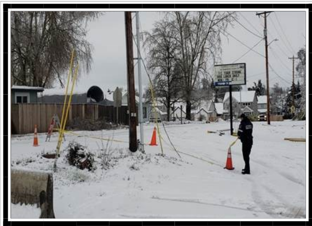
3rd St. And Polk St. (Downed wires)
