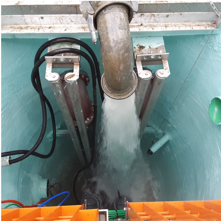
Hawn Creek Pumps being tested with a temp recirc pipe on 11/29/2022
